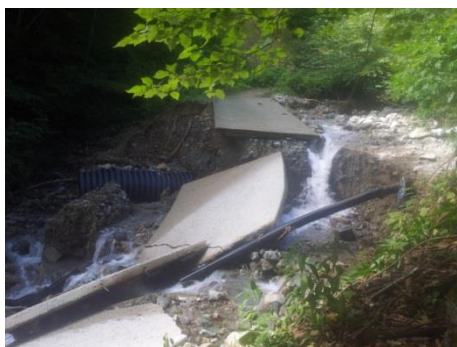
(導水管の被災状況)
