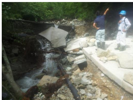
(導水管の被災状況)
