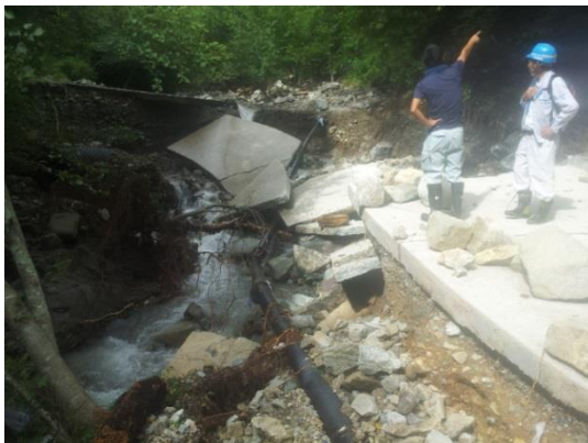
(導水管の被災状況)
